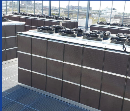
Equinix Datacenter - The Netherlands
