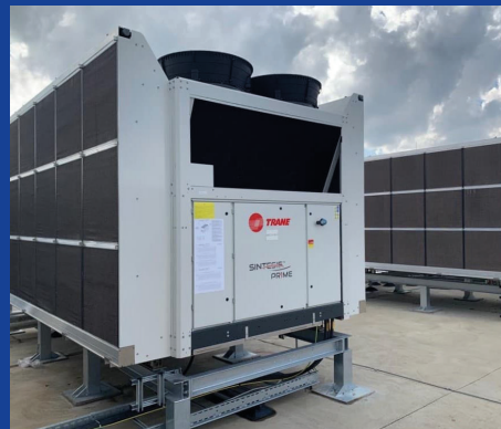
Equinix Datacenter - United Kingdom
